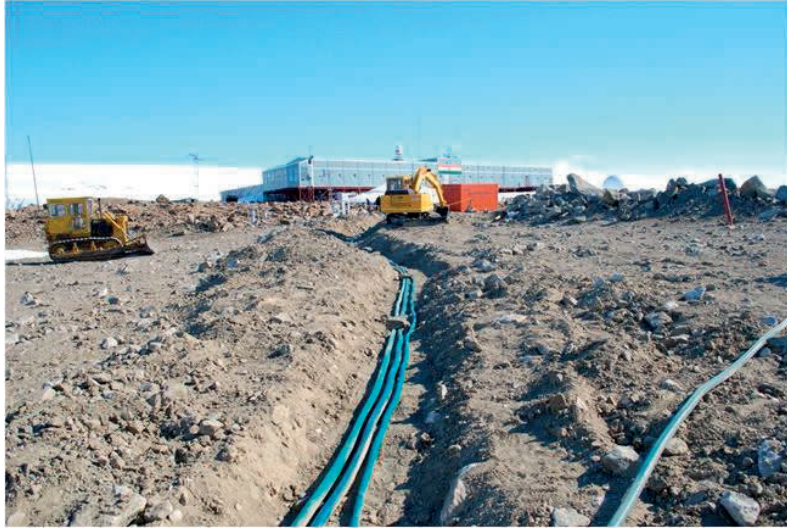
IT Cables running towards Maitri
