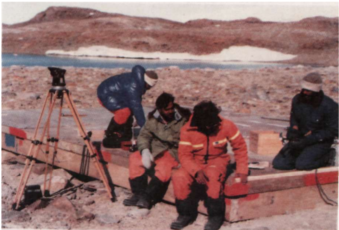
Fig. 6. Foundation of a cottage at Maitree station is ready for the erection of structure (Photograph: B.B. Bhattacharya)
