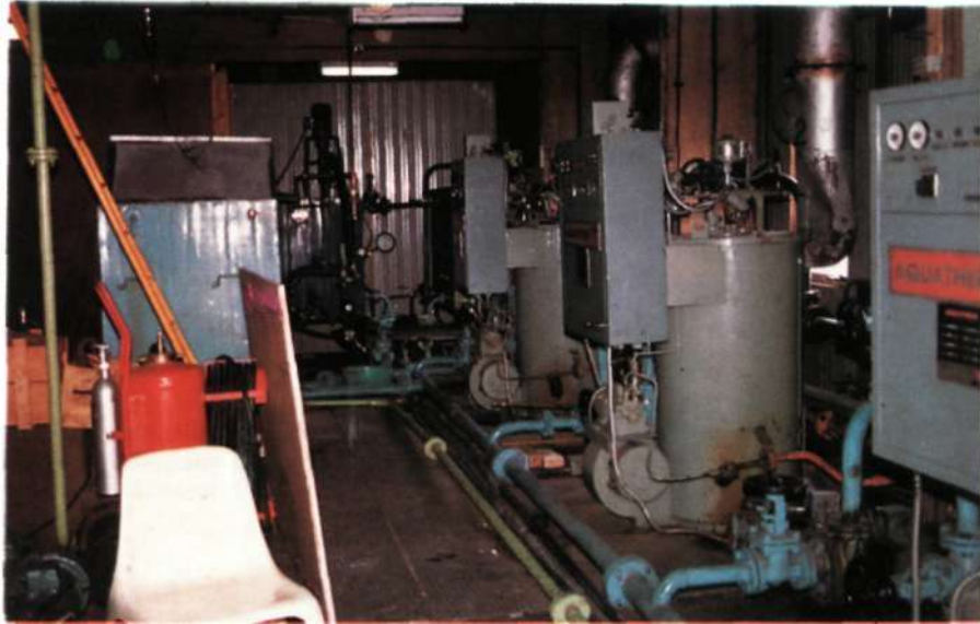
Fig. 1. Aviation fuel fired, hot water boilers in the Boiler room of Maitri station.
