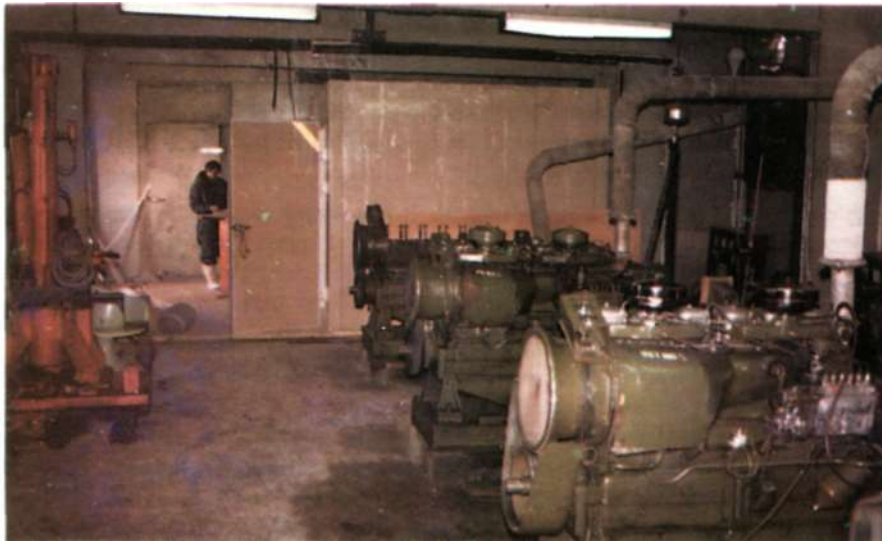
Fig.3. 62.5 KVA Ruston gensets inside the Generator Block. The walk-in cold room is also seen at the far end.
