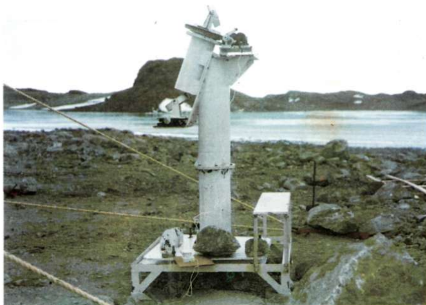
3. Sun tracker installed outside the Laser hut in Maitri
