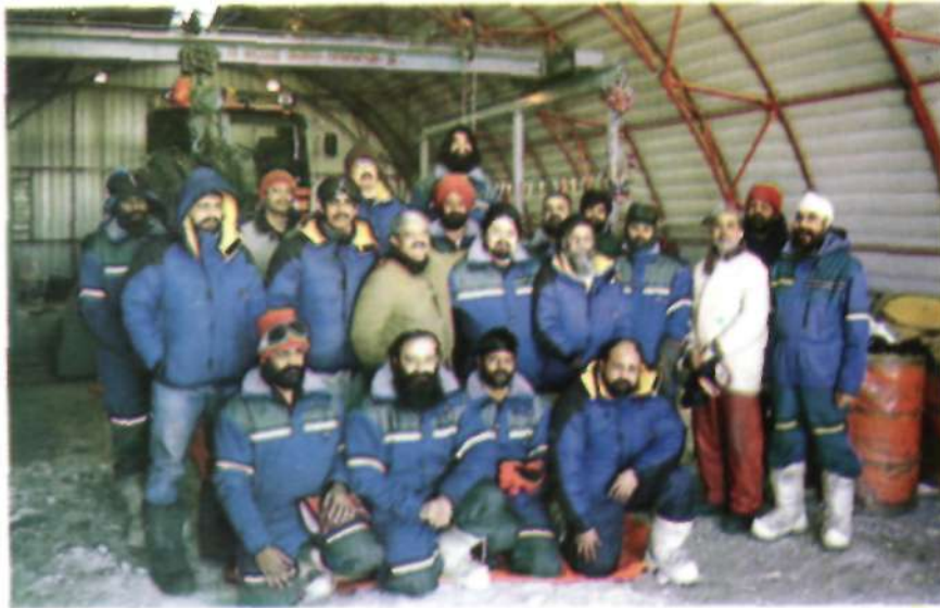
5. Successful completion of the Gantry-erection and Winch-installation by Army members (Photo: V.D.Abraham)
