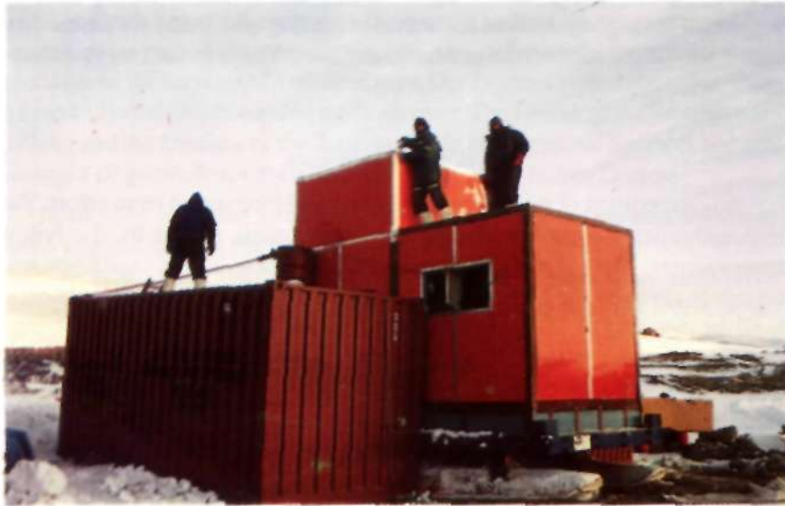
1. Construction of Ice-Core Drill Shelter by the Army members (Photo: Rajesh Bhat)
