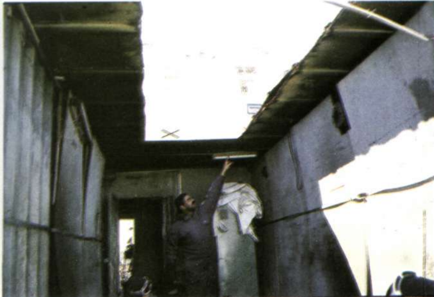
Installation of two new 125 KVA generators by cutting the roof of the containers.
