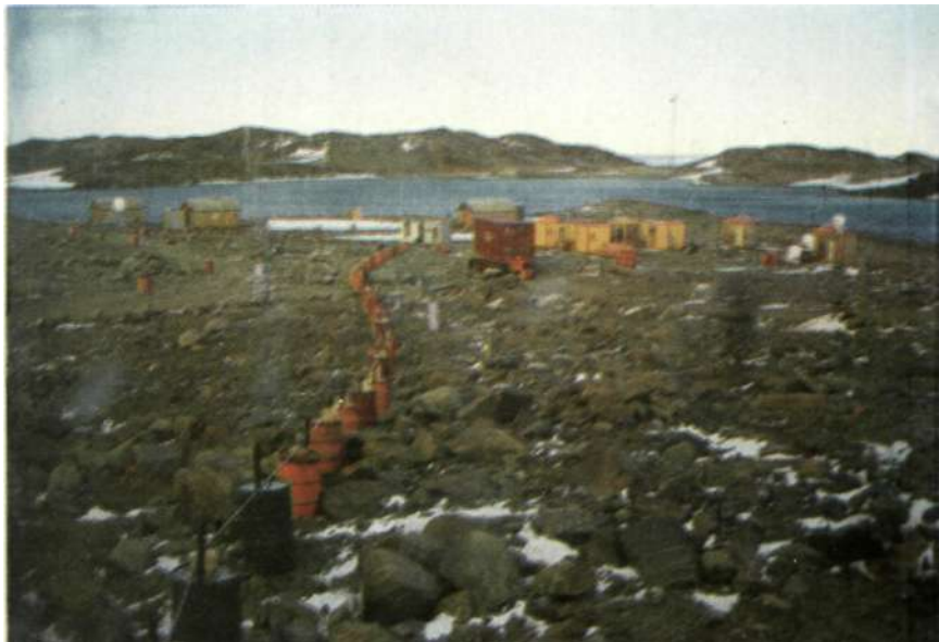
Laying out a new water pipe line for the summer camp at Maitri.
