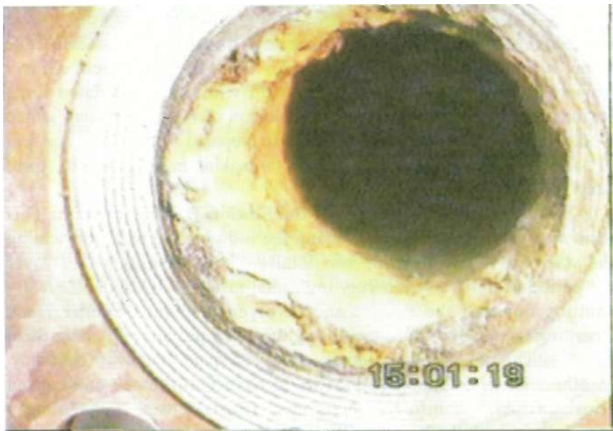
Fig. 7: The corroded old hot water pipe.
