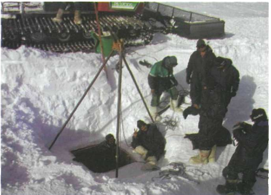
Photo-5: Retrieval of Ice Core from the buried building by a 'human-chain'
