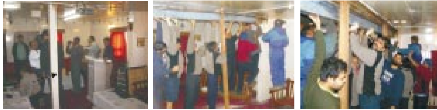
Fig. 9 : View of Maitri lounge with the obstructing pillar, removal of the pillar and re-strengthening by iron beam
