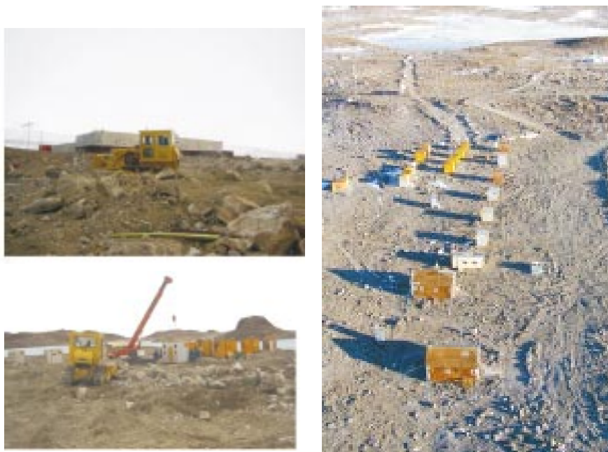
Fig. 23 : Levelling of summer camp area, making of utility pathways and repositioning of summer huts
