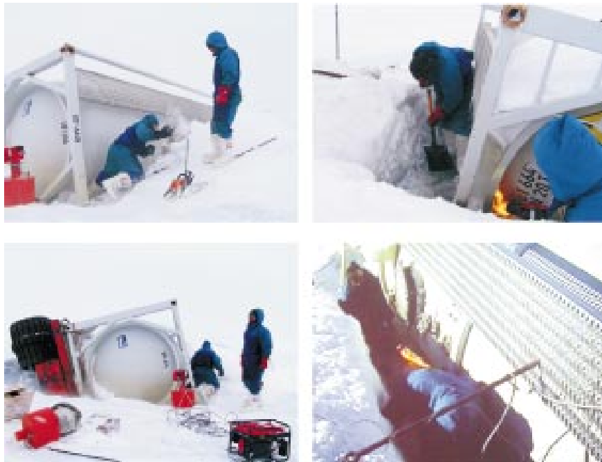
Fig. 6 : Various stages of attempt to release the tanker and trailer using electrical burners for melting surrounding ice
