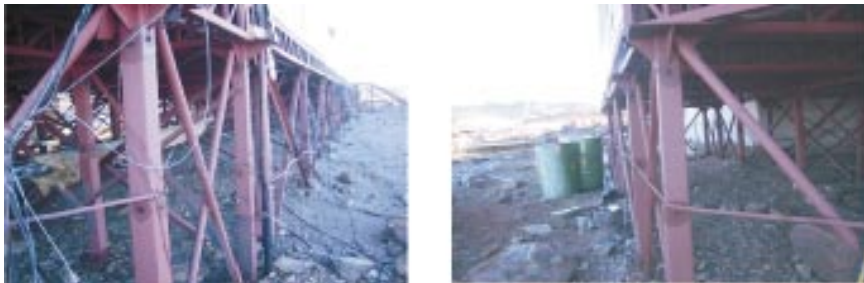
Fig. 25 : Removal of redundant, old communication and electrical cables from the structures of Maitri
